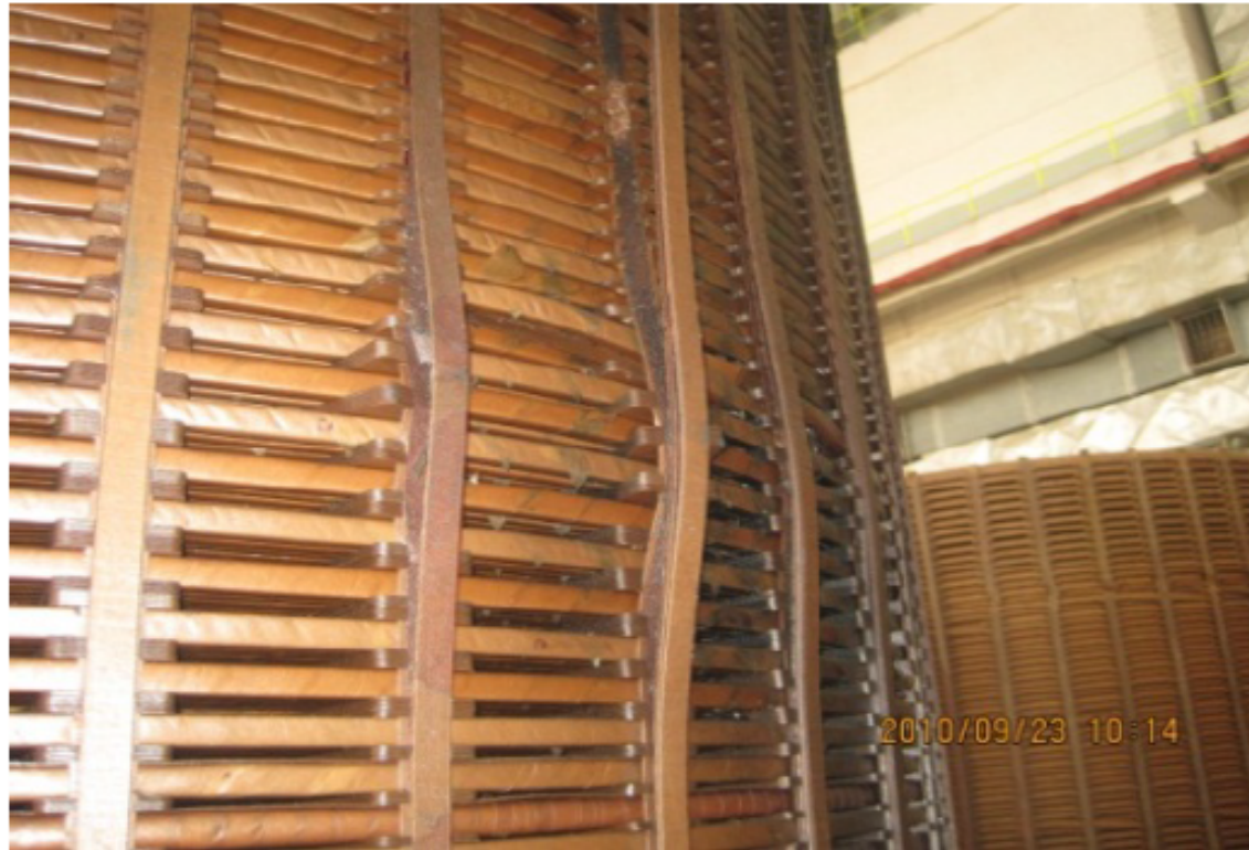
Figure 4 – Transformer winding buckling fault [2]
